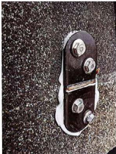
Figure 4b. Mount failure mode.
