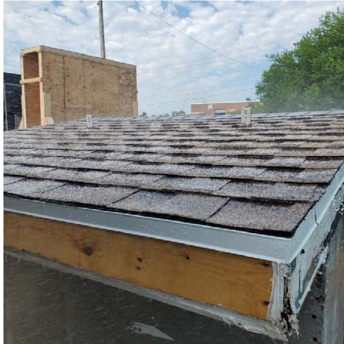
Photo No. 3 35 MPH Top Side
