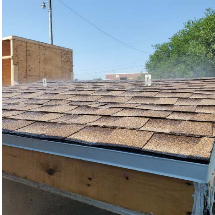
Photo No. 9 110 MPH Top Side
