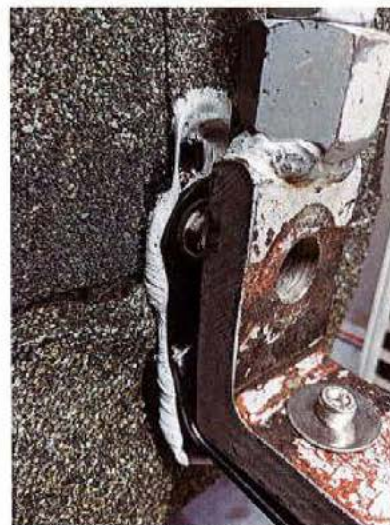
Figure 4c. Bolt failure mode.
