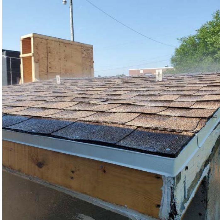
Photo No. 5 70 MPH Top Side
