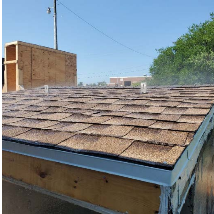
Photo No. 7 90 MPH Top side
