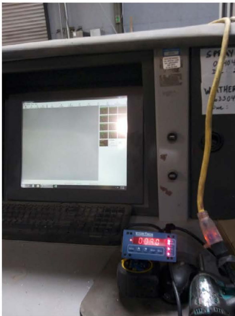
Photo No. 5 Instrumentation
