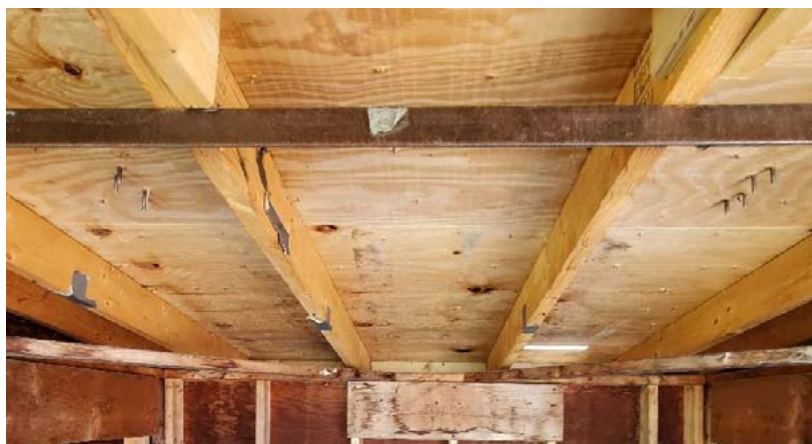
Photo No. 12 Post Test Underside
