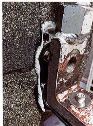
Figure 4c. Bolt failure mode.
